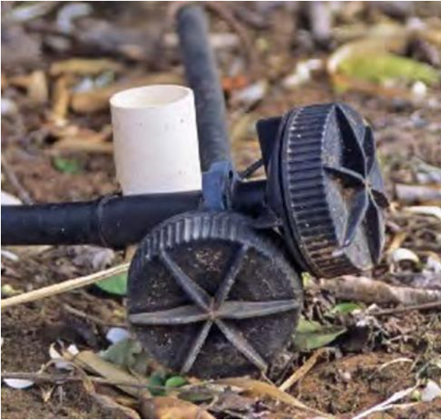
Figure 3. Automatic flush valves
