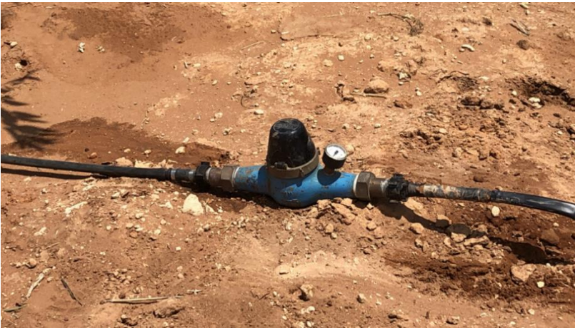
Figure 11. In-line flow meter installed in a lateral. Photo: Mark Skewes
