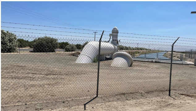
Ground Water Recharge Pump Terranova Ranch USA
